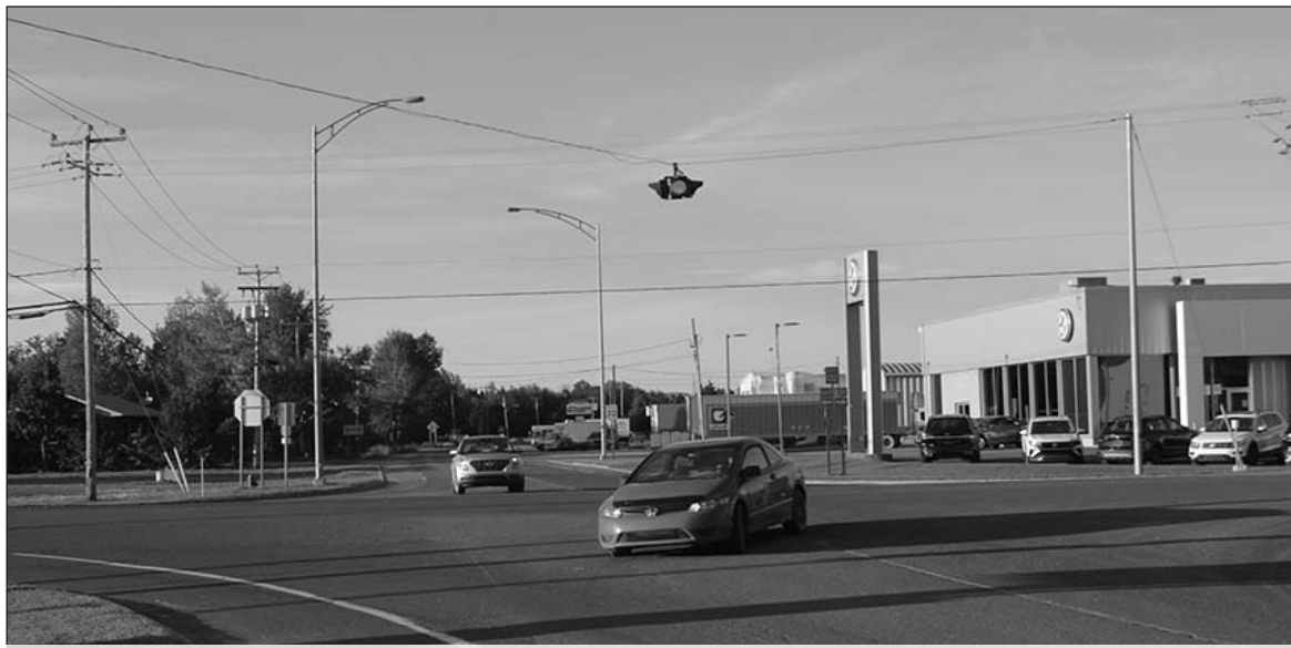
The project to install traffic lights at the intersection of Highway 132 and Saint-Edgar Road was approved at the end of spring 2021 (photo) but only started over the last weeks.
