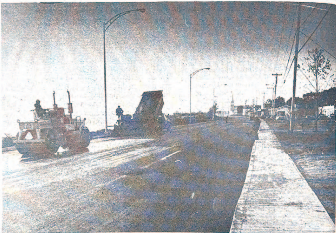
Caplan residents breathe a sigh of relief as construction draws to an end on their section of Route 132 this week. Those forced to travel through Caplan on a regular basis also had their fair share of bumps and grinds since the construction began this spring. It's rumoured that New Carlisle will be next to face a similar predicament.
